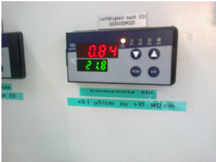
The general plant
