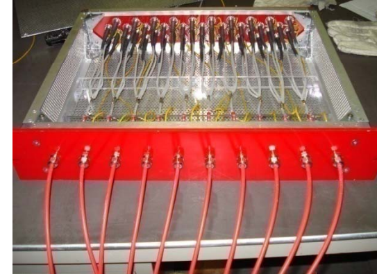
Input Side of Distribution Box
