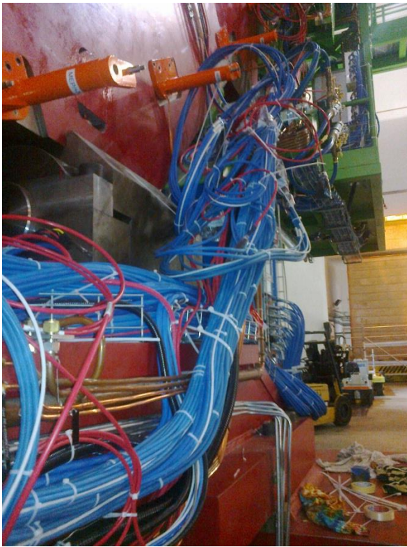
Dense cabling in front of the Near Pivot.
